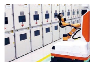
Robotic High-voltage Switchgear Operation
